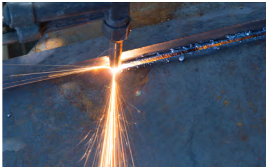
Hot surfaces during metal cutting
